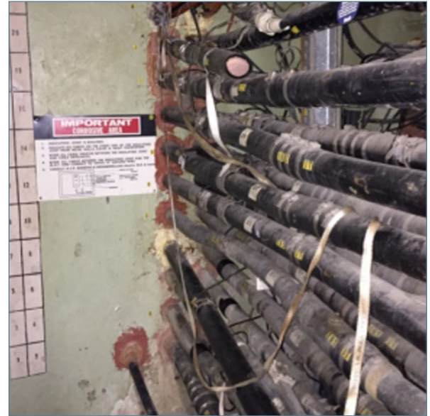
Figure 3: Cable vault – Removing copper through migration opens duct space. The many copper cables shown here can be replaced by fiber cables (wrapped in orange), that take up much less duct capacity.
