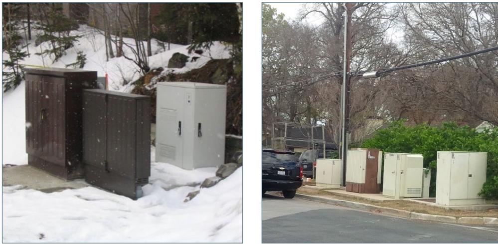
Figure 5: Fewer cabinets, less power – Fiber uses less space and no power with a single, smaller passive FDH cabinet replacing two brown DSLAM cabinets, making it green and aesthetically appealing.
